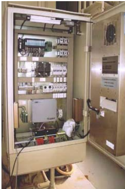
PD Monitoring System installed
